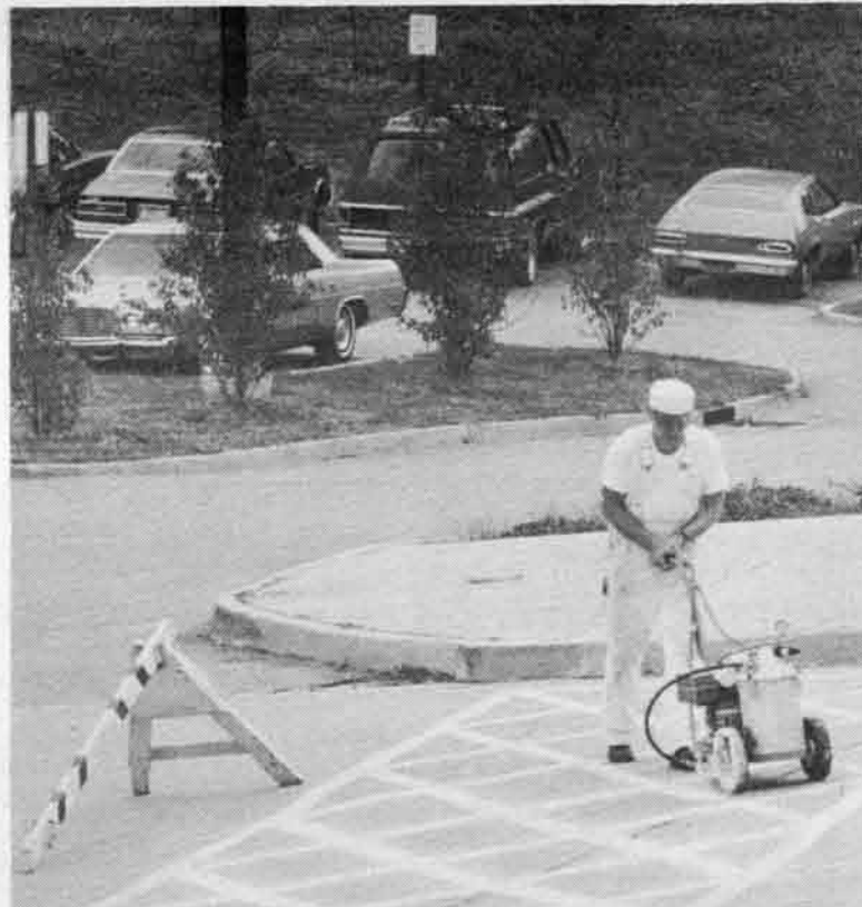
WALK THE LINE: A University workman repaints the crosswalk lines between Woods Hall and J.C. Penney last week. [Photo by Dale Nelson].
